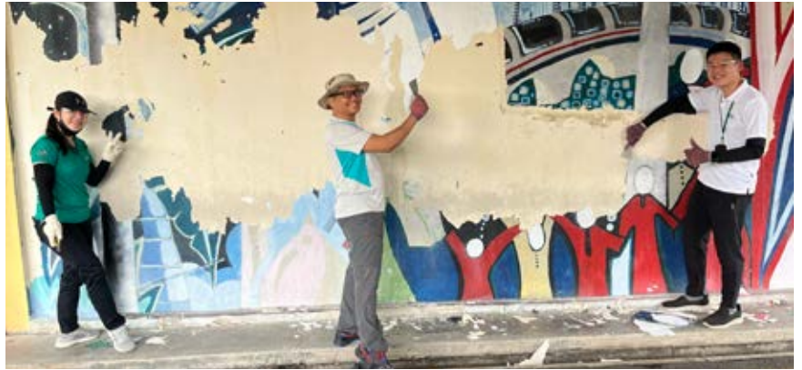
Before given a fresh coat of paint, the old layers had to be scraped off the walls.
